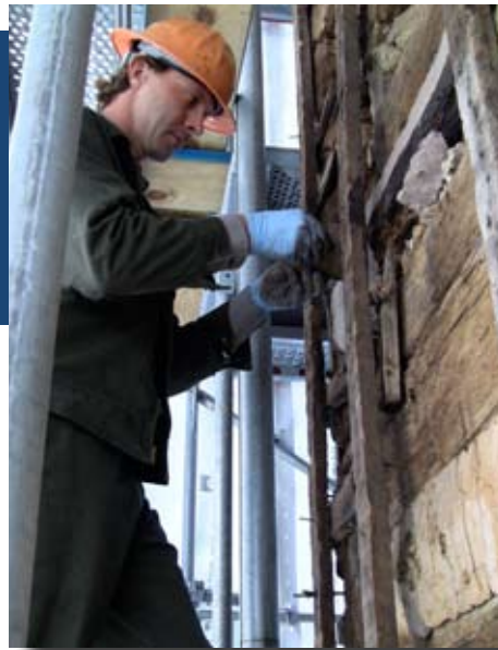
Travis applies the epoxy into the cavity where rotted wood has been removed.
