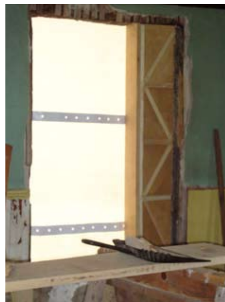
The Maintenance Division has been reconstructing the window casings to their 1862 dimensions.
