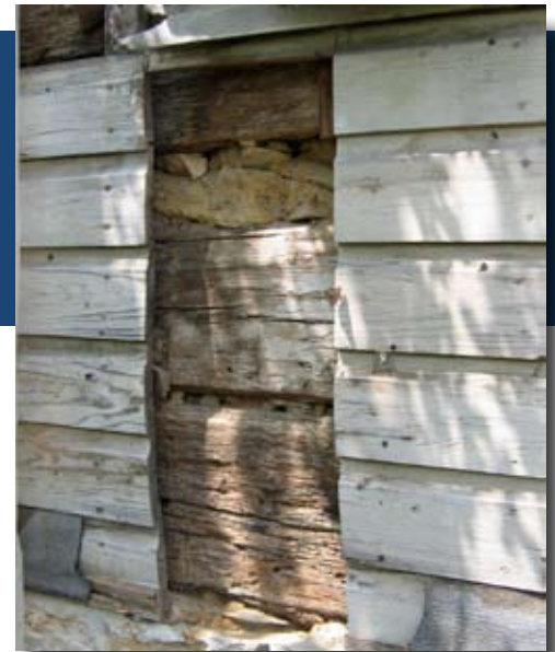
Removal of the modern siding reveals the original log construction of the house.
